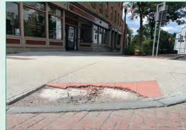
Above: Existing curb ramp in need of replacement
